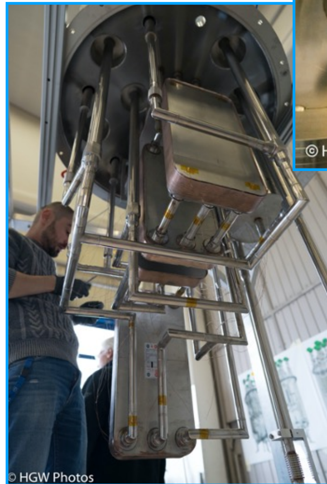
In-house fabrication of the gas handling system
