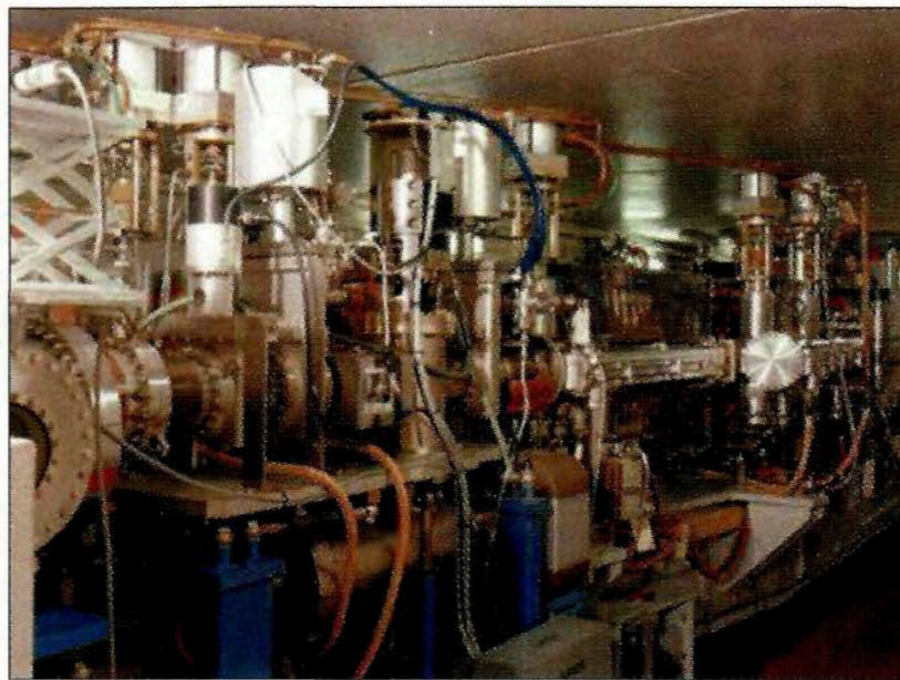
Part of the ALS storage ring at the Lawrence Berkeley National Laboratory. Frequency mapping was first applied to measured rather than simulated electron trajectories at the ALS.
