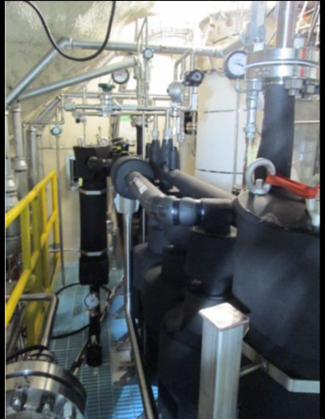
Scintillator purification plant underground
